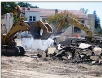
Marin CCD Kentfield campus demolition for New Science & Math Central Plant GC: Lathrop CM: Swinerton Management & Consulting
