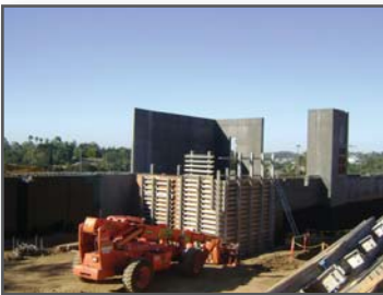
Palomar CCD Industrial Technical Center GC: James Corporation of California CM: Gilbane
